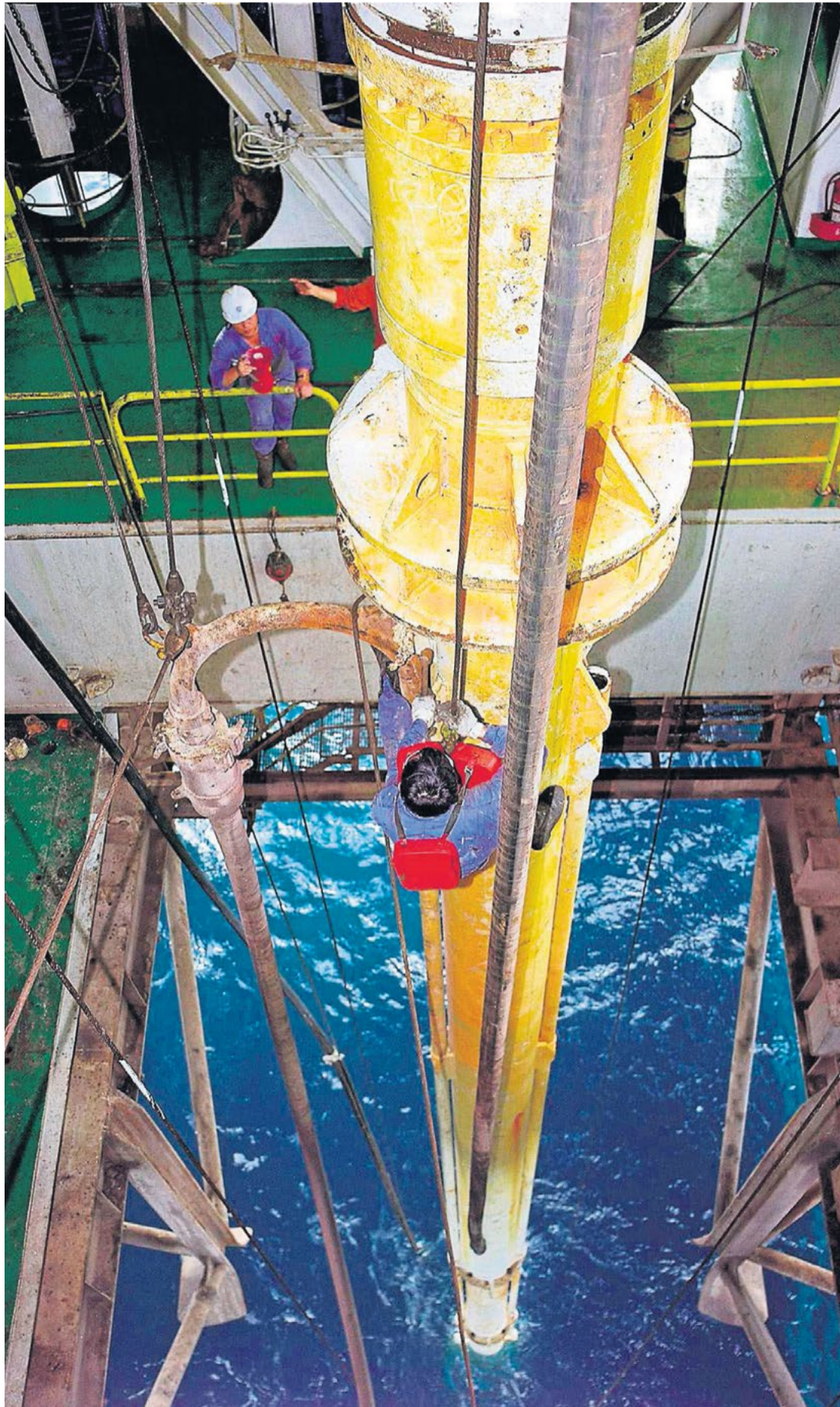
Drilling ahead: workers on a CNOOC platform in the South China Sea Photo: REUTERS/SCANPIX
